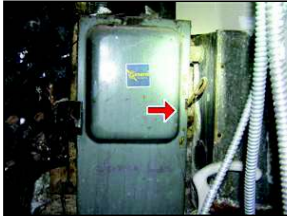
8.9 Picture 1 Main shut off switch
