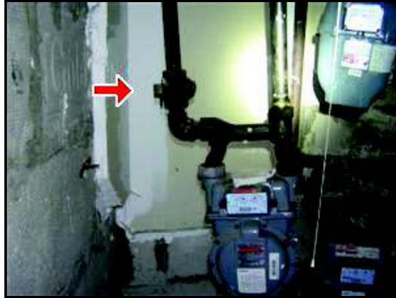
7.5 Picture 1 Hole house gas valve
