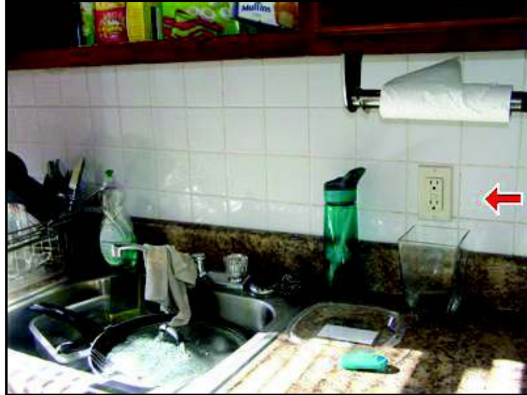
8.5 Picture 1 GFCI outlets in 2nd floor kitchen.
