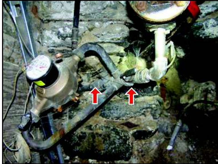
7.3 Picture 1 Potable water shut off valves
